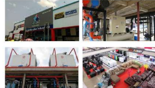
Design and Install Air-Conditioning System Water Cooled Chiller 206.9 Ton(2)
