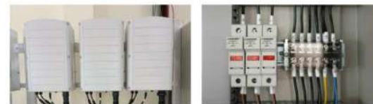
Solar cell System 147 kWp
