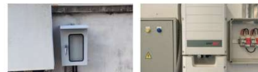
Solar cell System 35.2 kWp
