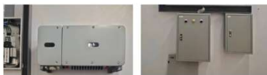
Solarcell System 61.6 kWp
