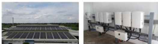
Solar cell System 185 kWp
