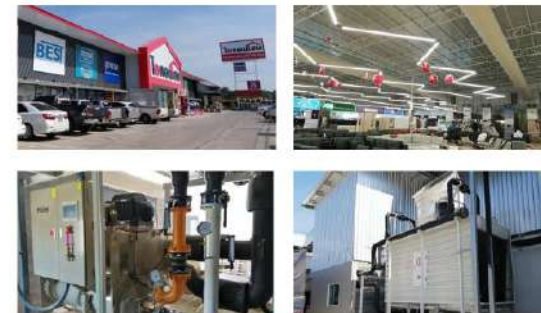
Design and Install Air-Conditioning System Water Cooled Chiller Magnetic Bearing 142 Ton
