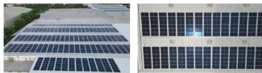
Solar cell System 594 kWp
