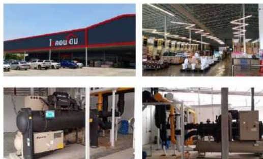
Design and Install Air-Conditioning System Water Cooled Magnetic bearing Chiller 150 Ton
