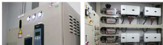
Solar cell System 264 kWp
